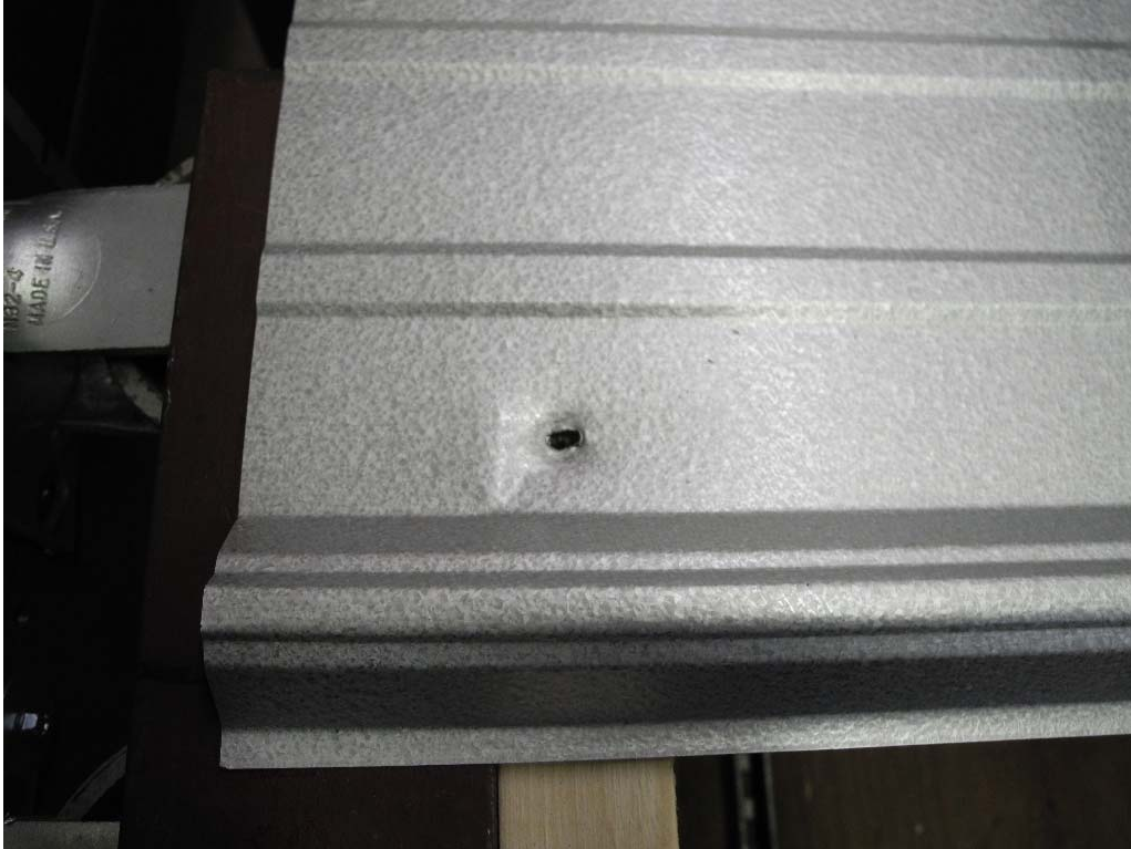
PHOTO 5 View of panel slotting at fastener near the roller support in Test #1. (DSCN0015)
