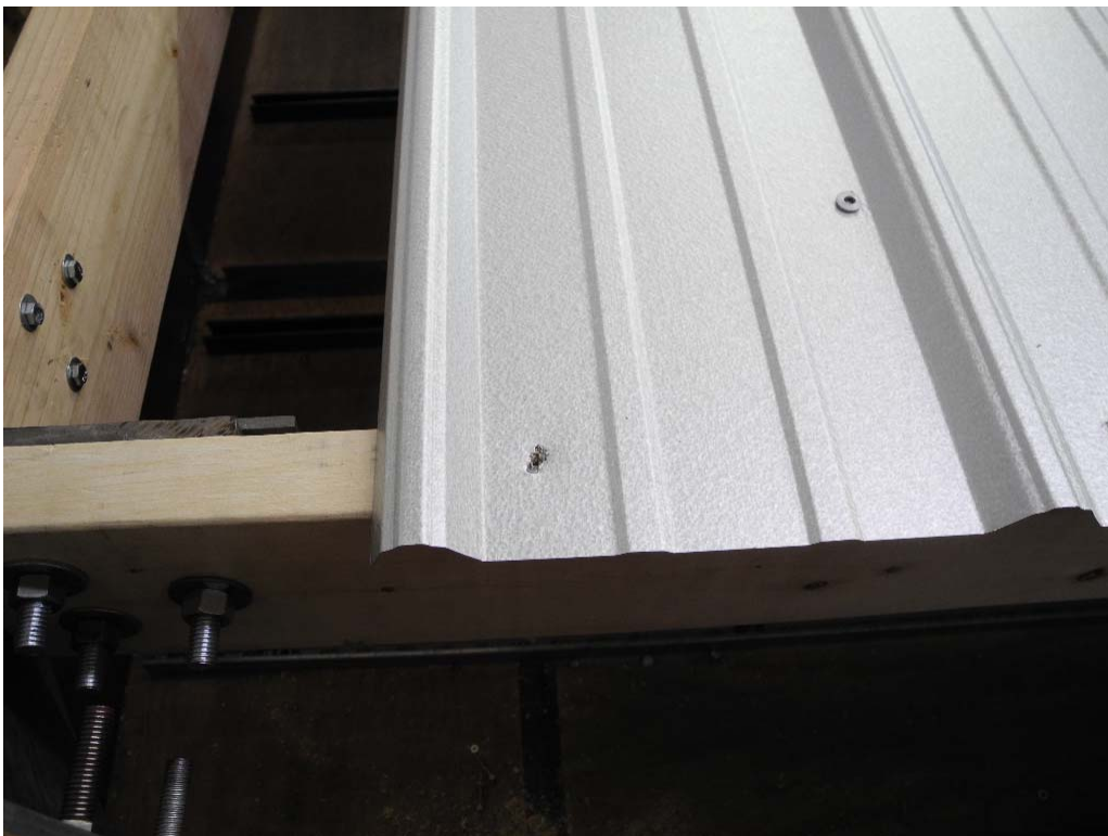
PHOTO 6 View of panel slotting at fastener near the pinned support in Test #2. (DSCN0021)
